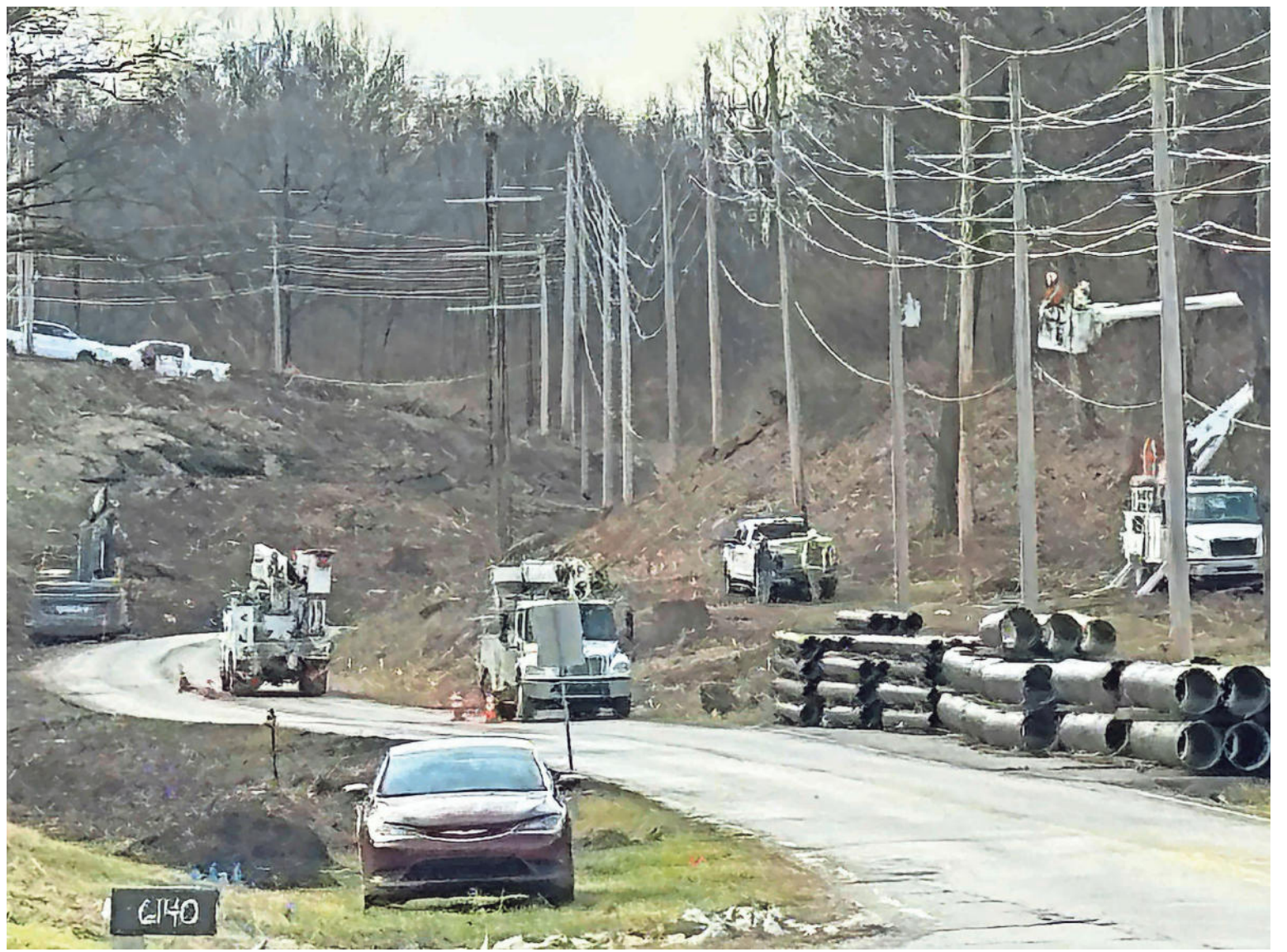
Crews have been moving utility poles as part of Kansas City Public Works’ project to widen Lee’s Summit Road between Lakewood Boulevard and Anderson Drive, just south of Independence. The road, seen here from the entrance to the Space Center Summit caves, has been closed since August 2023 and will remain closed until the fall of 2025. [Mike Genet/The Examiner]
